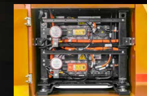
Battery and motor radiator
